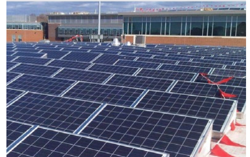
Solar Panels on top of PEC. Photo by Bithenergy
